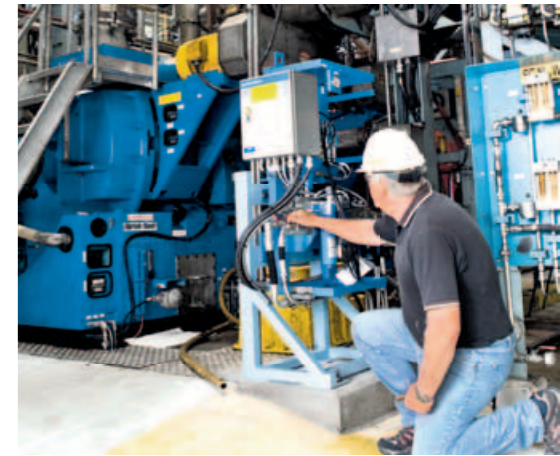
▲ Port Alberni was the first in North America to install the ANDRITZ Refiner Commander. The plate positioning sensors and dual servo split the Twin refiner’s hydraulics into two separate loops which are controlled independently. “The result is less clashing, better performance, and phenomenal plate life,” says Sandy Shearer, CTMP #1 Operator.
