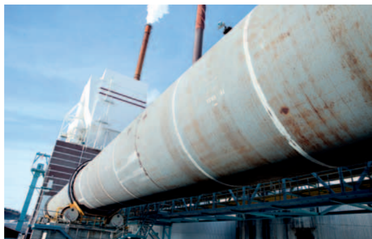
Pellets from SCA’s BioNorr plant are ground at the mill to become fuel for the ANDRITZ kiln. ▶
