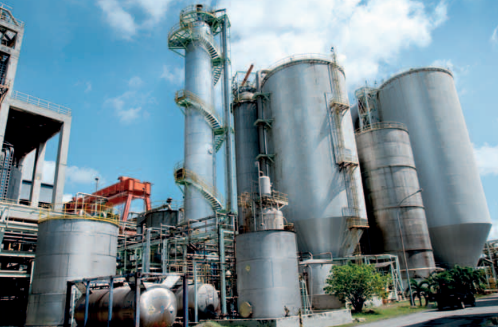
◀ A new two-stage oxygen delignification system from ANDRITZ (left and below) significantly reduced the Kappa number into the bleach plant and eliminated the bleaching bottleneck without jeopardizing pulp brightness.
