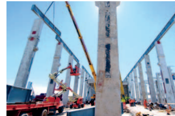
▲ ANDRITZ is the main technology supplier for the entire Montes del Plata mill – with a scope covering the woodyard, fiberline, pulp drying/baling plant, chemical recovery block, white liquor plant, and power island. Shown here is the fiberline building taking shape.
