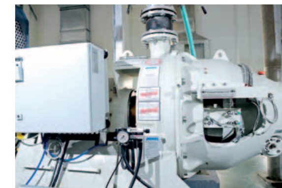
▲ ANDRITZ supplied the stock preparation (two virgin fiber lines and a broke line), approach flow, and fiber recovery systems. Shown is the LC refiner which helps optimize the virgin fibers to improve paper quality.
