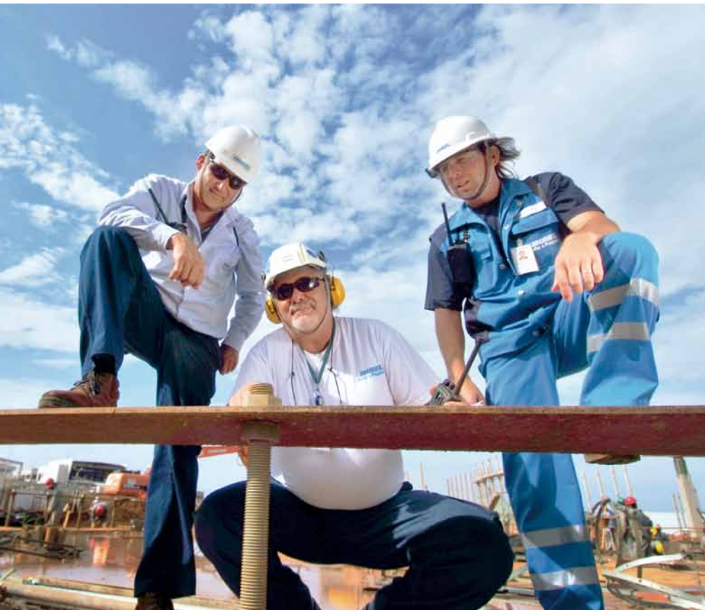
The largest digester in the world. ANDRITZ's Gustavo Guastti, Materials Coordinator (left); Rafael Batistela, Fiberline Erection Manager (center); and Silas Navarro, Fiberline Mechanical Supervisor are standing on the foundation of the 5,100 adm/d ANDRITZ continuous digester. ▼
