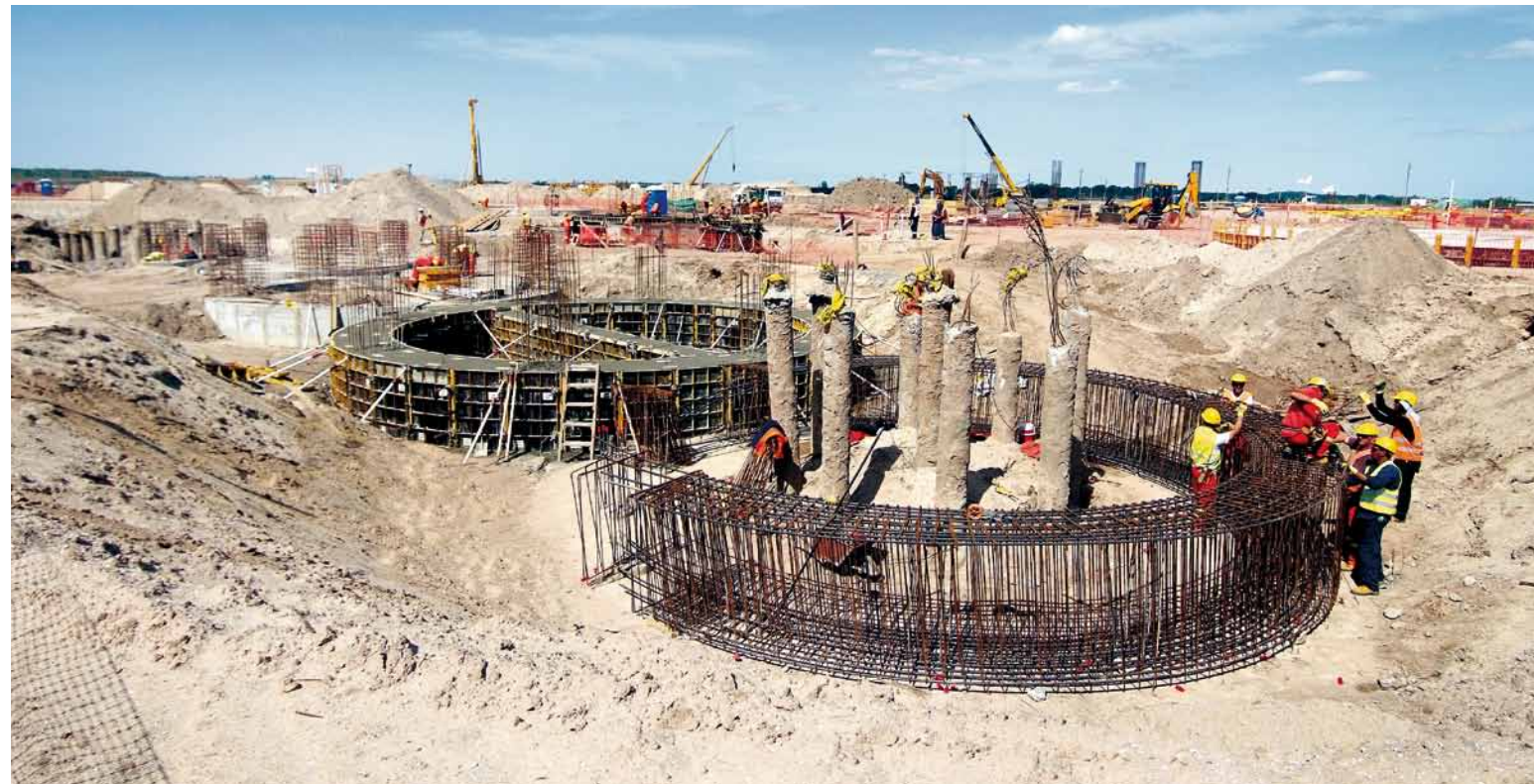
Civil construction crews pour foundations for recausticizing tanks in the white liquor plant. ▼
