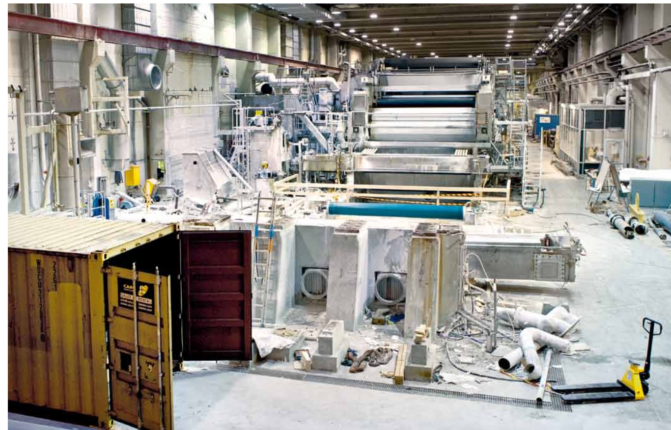
▼ A view of the machine room at UPM Kymi's mill where the machine is being dismantled and inspected. ▼
