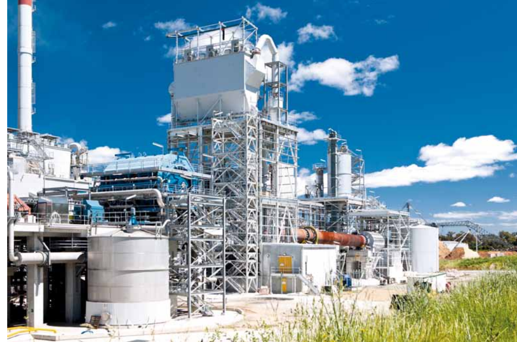
▲ A second white liquor plant (shown above) from ANDRITZ was part of the expansion.
