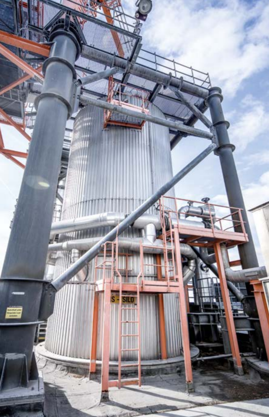
Modified HELP™ discharge with center steaming provides excellent impregnation result.
