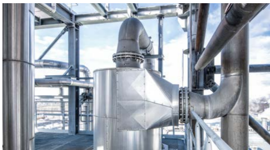
New gas handling system ensures safety and odour-free operation of the chip bin.
