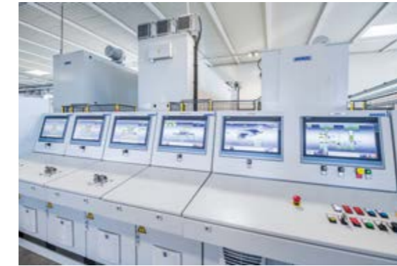
Monitoring system to guarantee smooth operation and enhance production
