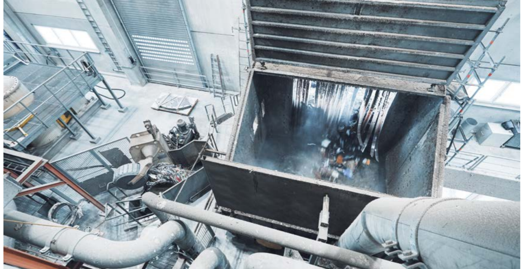
The former grinding facility was converted to an RCF line with a capacity of 1,350 tons per day. An ANDRITZ FibreSolve FSR pulper complete with disposal system ensures optimum pulping of the raw material.
