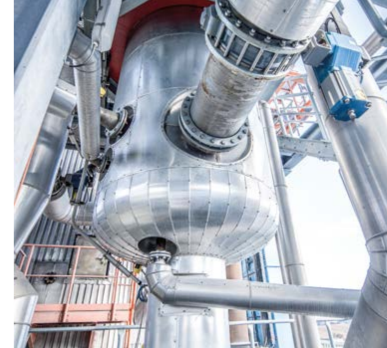
Vapor reboiler generates fresh steam utilizing the energy of hot black liquor (Flash steam) and fractionates the flash steam condensate to turpentine rich and clean condensates.
