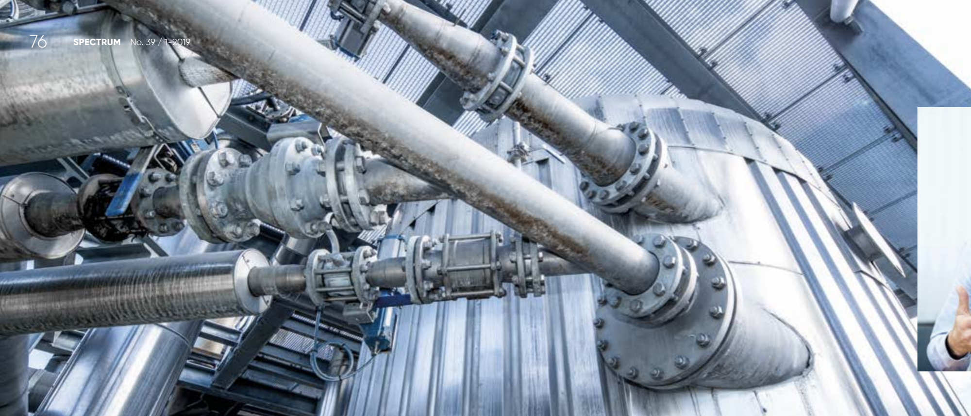
Black liquor is flashed in new ANDRITZ efficient flash tank utilizing FlashLance™-technology.
