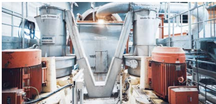
ANDRITZ ModuScreen TD coarse screen as part of the stock preparation plant
